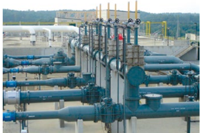
30", 36" & 42" Solid SS Bonneted Knife Gates, 50 psi, Wastewater Treatment Plant Gwinnett County, GA
